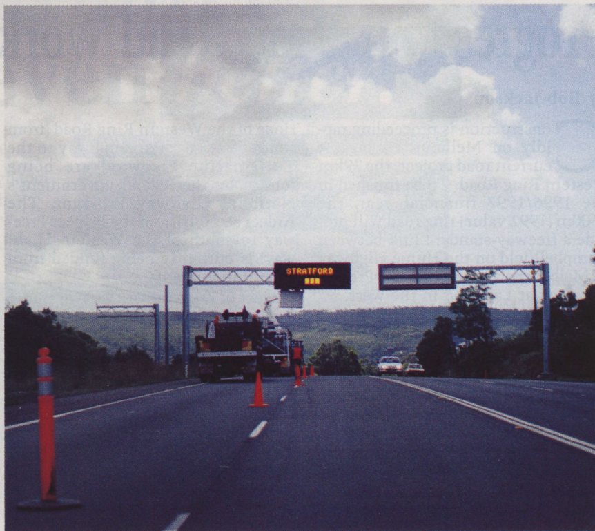
A Stratford Traffic fibre optic sign being installed on the F6 Motorway near Wollongong
